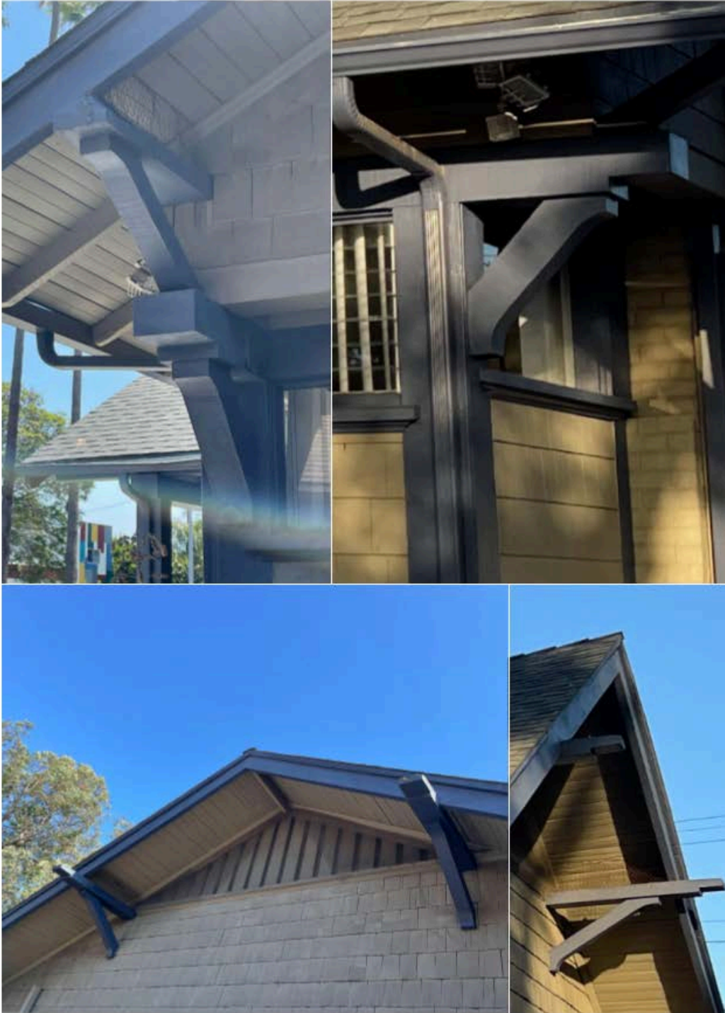
Webster's signature knee-braces with integral feet. Source: photo taken by nomination preparer, 2022
