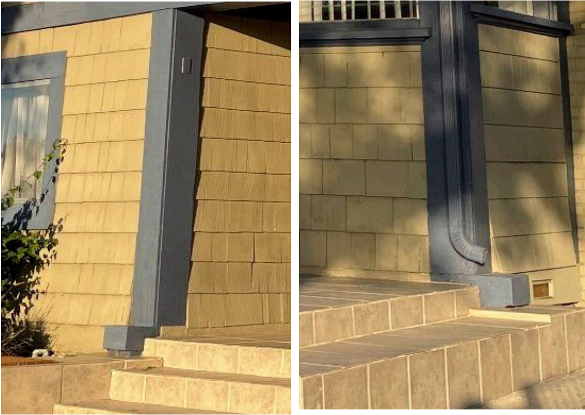
Examples of the faux mudsills as part of the larger faux post-and-beam structure, lending the appearance of a medieval Japanese structure to the bungalow. Photo taken by nomination preparers.
