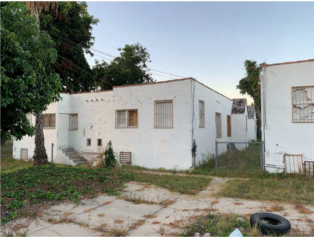
South facade of southwestern unit, facing north. Source: Lindsay Mulcahy/ L.A. Conservancy, 2023.
