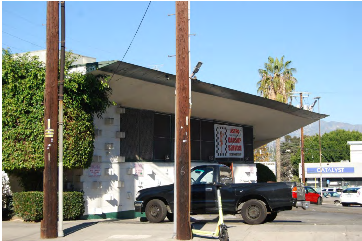
Astro Family Restaurant, roof overhang at rear, 2306 Fletcher Drive, November 22, 2022 (Photograph by Charles J. Fisher)
