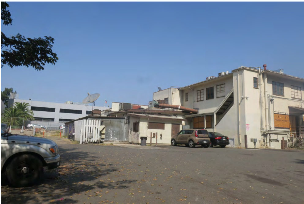
South and east façades of 2-story addition and refrigeration plant, view northwest (ARG, 2021).
