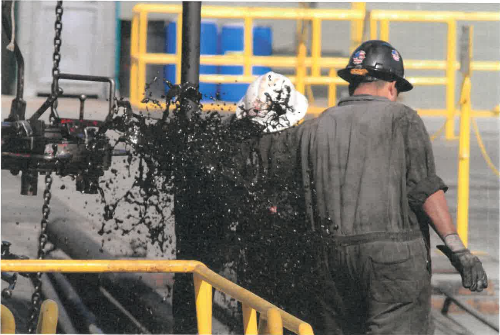
Figure 26 - Oil splashes bare armed workers who tried to suppress the oil burst by wrapping the pipe with a plastic trash bag (4/15/2021)
