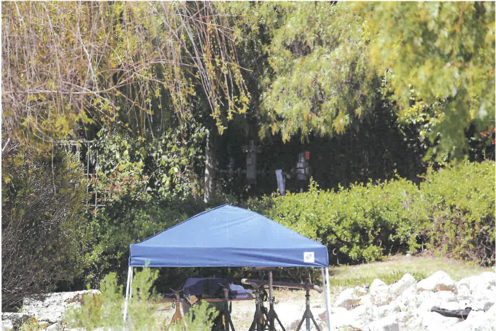
Figure 8 - Tents, tools, and pipes were let out overnight and over the weekend. The new meter set assembly is visible in the background (3/27/2021)
