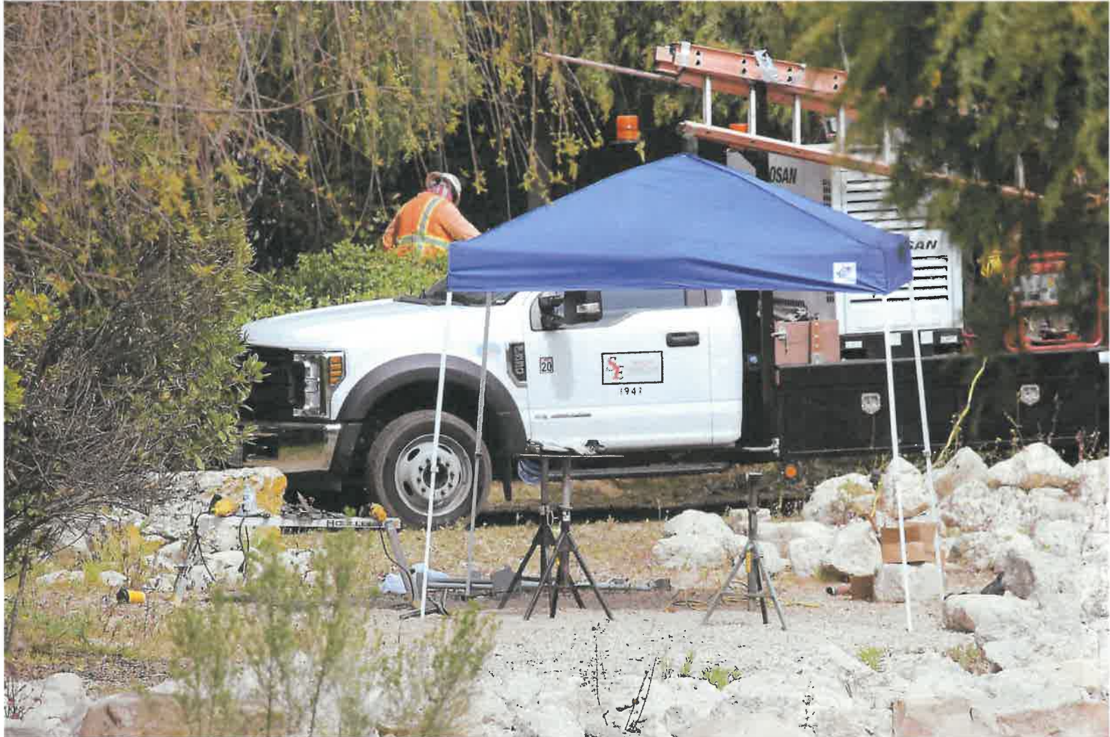
Figure 2 - Truck parked in the south side of the lease with a massive generator and other tools. Pipe-fitter work station (3/25/2021)
