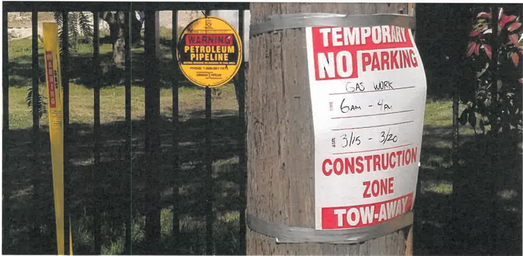
Figure 6 - Fake NO PARKING / TOW-AWAY zone set up by Murphy workers (3/16/2021)
