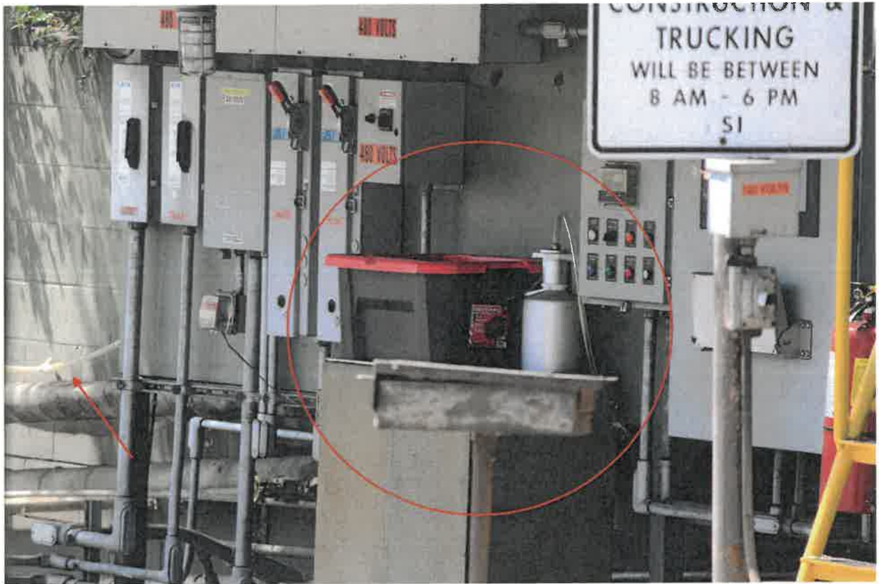
Photo 5: The silver device appears to be a diffuser for dispersing odor counteractant. A clear plastic tube emerges from the top, runs under the shelter and then along the wall shared with the AIDS Healthcare Foundation. The device appears to be connected to the black plastic bin by a white tube.
