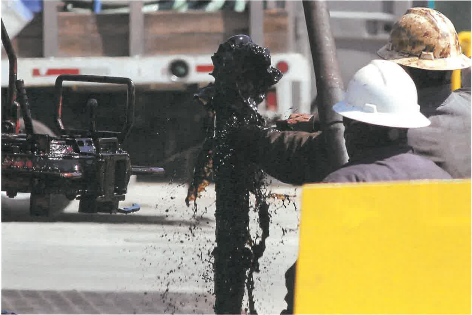
Figure 24 - A barehanded worker tries to stop the flow (3/17/2021)
