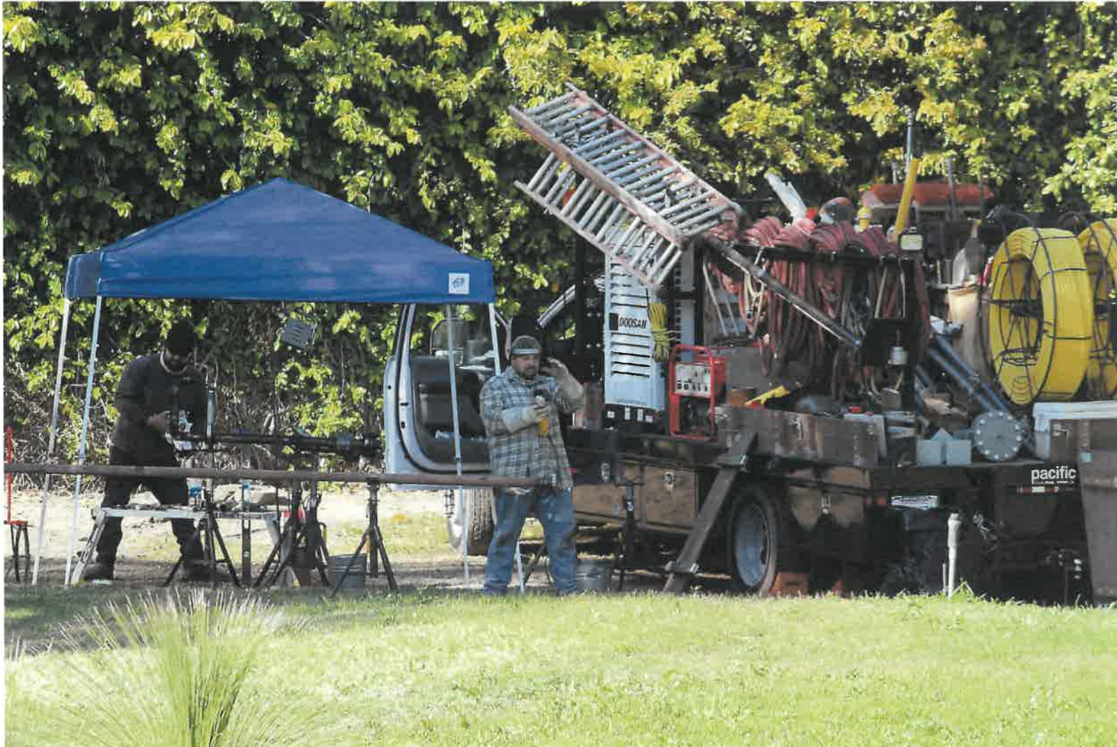
Figure 3 - Trucks and tents in the parkland. Pipe fitters and welders build a new gas meter set assembly (March 19, 2021)
