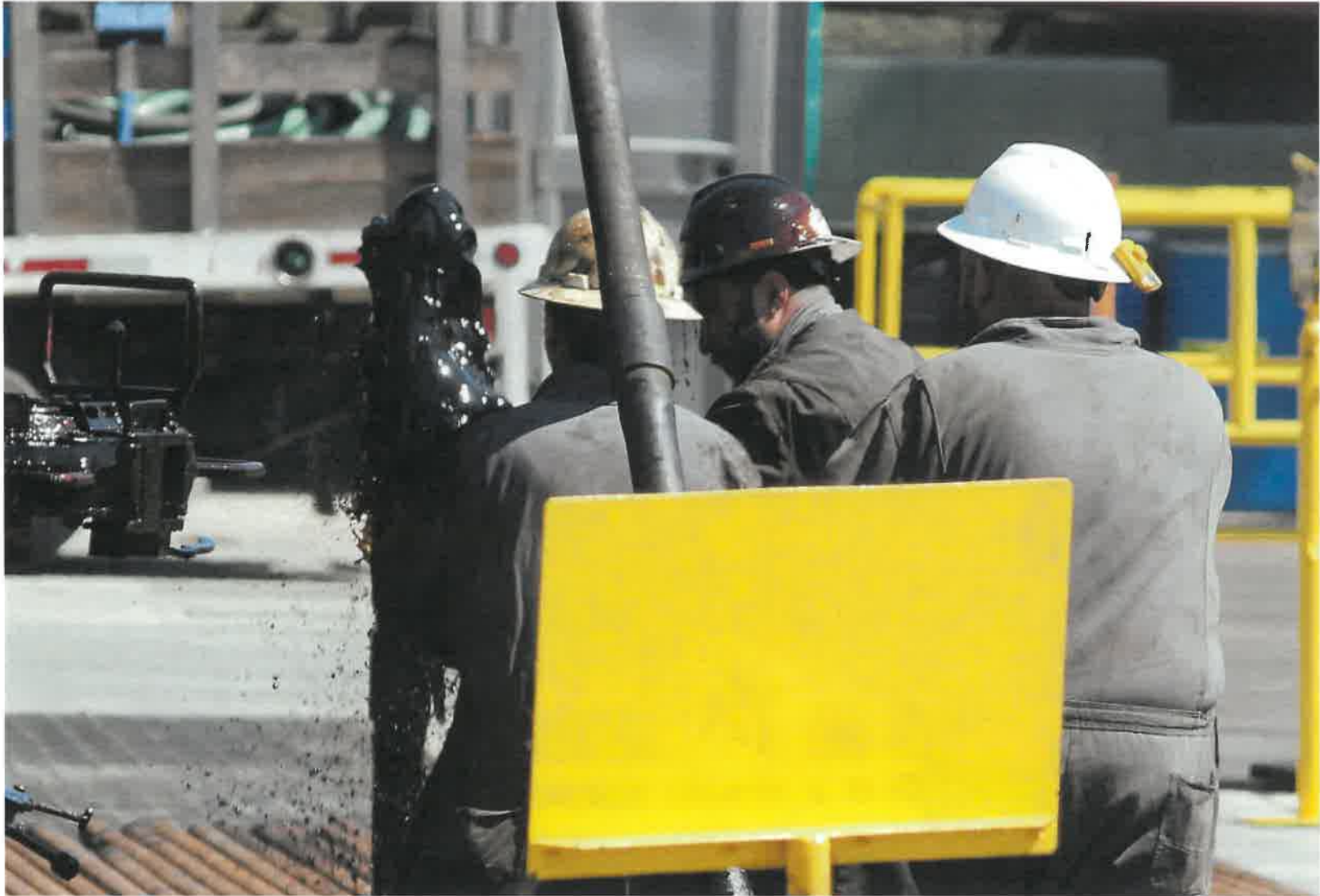
Figure 25 - Oil drips from a hard hat as workers without PPE try to stop the flow of oil (3/17/2021)
