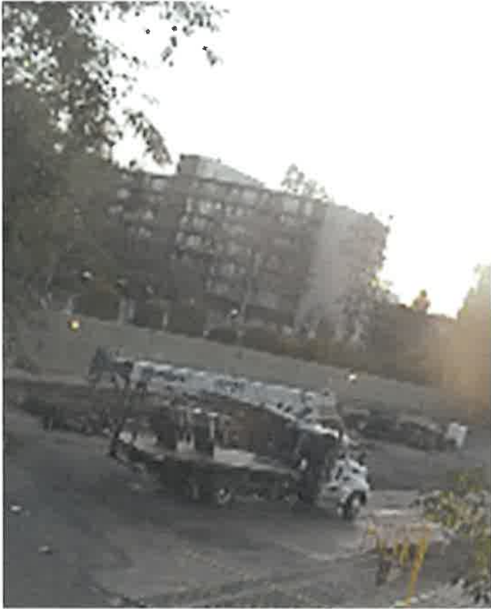
Figure 13 - On Saturday, April 10 at 6:45am a large truck with a mounted crane and large flatbed arrived on site carrying a tank
