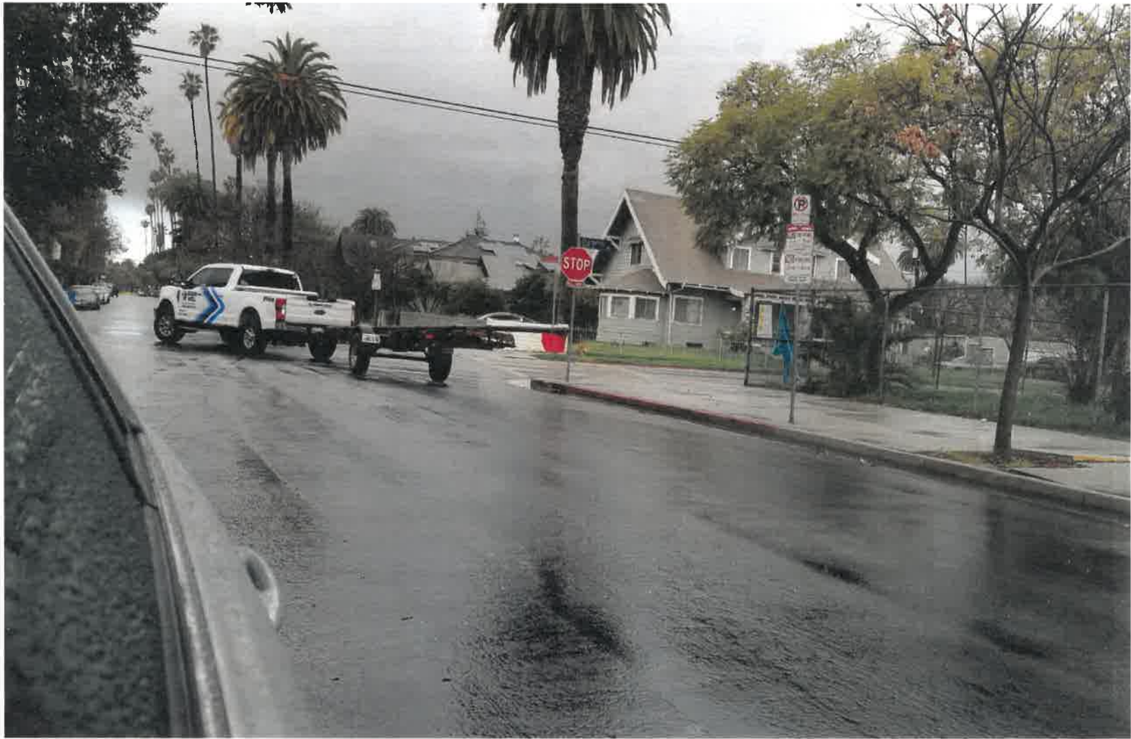
Figure 19 - Snow Well workers drive a large pipe past 24th St Elementary School and the Widney High School on 24th Street.
