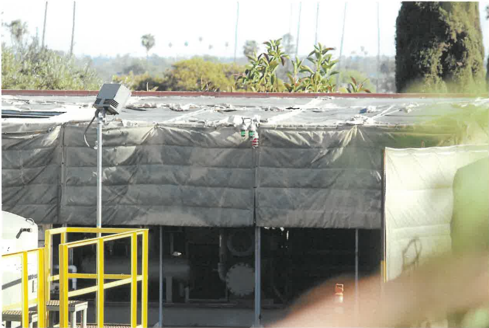
Figure 17 - Dilapidated sound blankets in the southwest corner of the drill site next to the AIDS Healthcare Foundation building.
