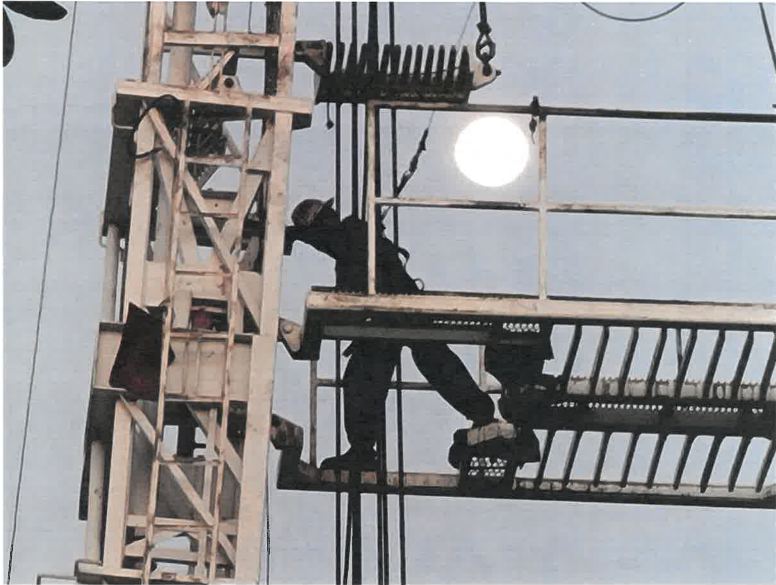
Figure 11: Moonlight bathes a worker high above the drill site on the workover perch (3/26/2021)
