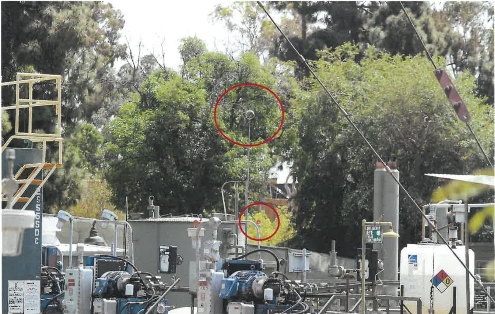
Figure 31 - Missing windsock as a red warning light flashes on the East wall (4/15/2021)
