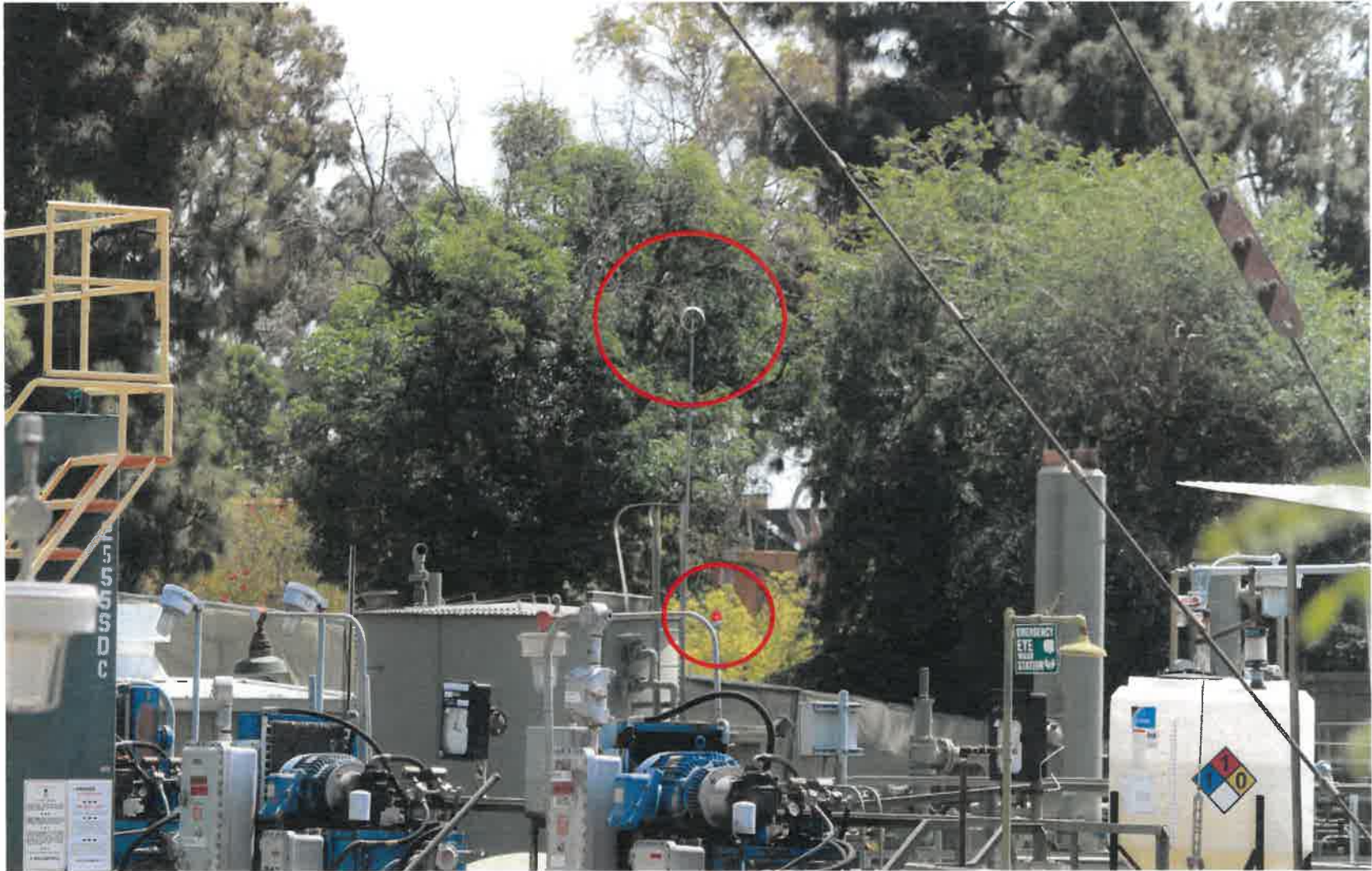
Figure 31 - Missing windsock as a red warning light flashes on the East wall (4/15/2021)
