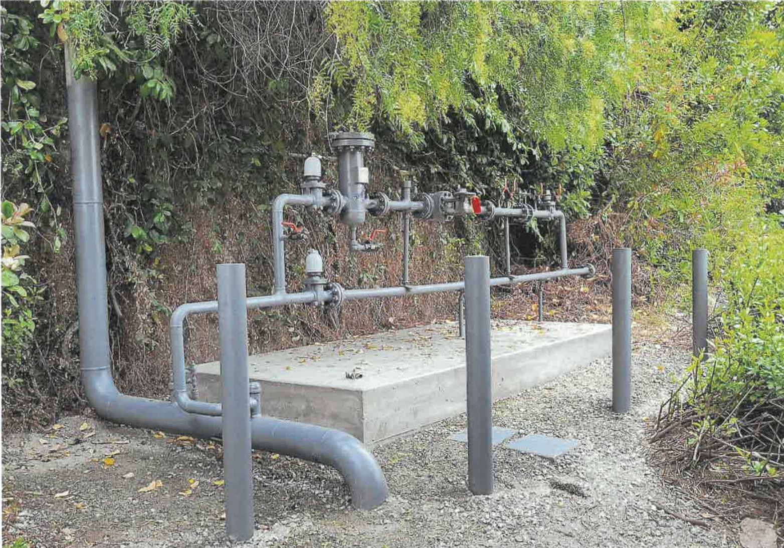
Figure 1 - New gas meter set assembly installed over concrete pad in the parkland (4/13/2021)
