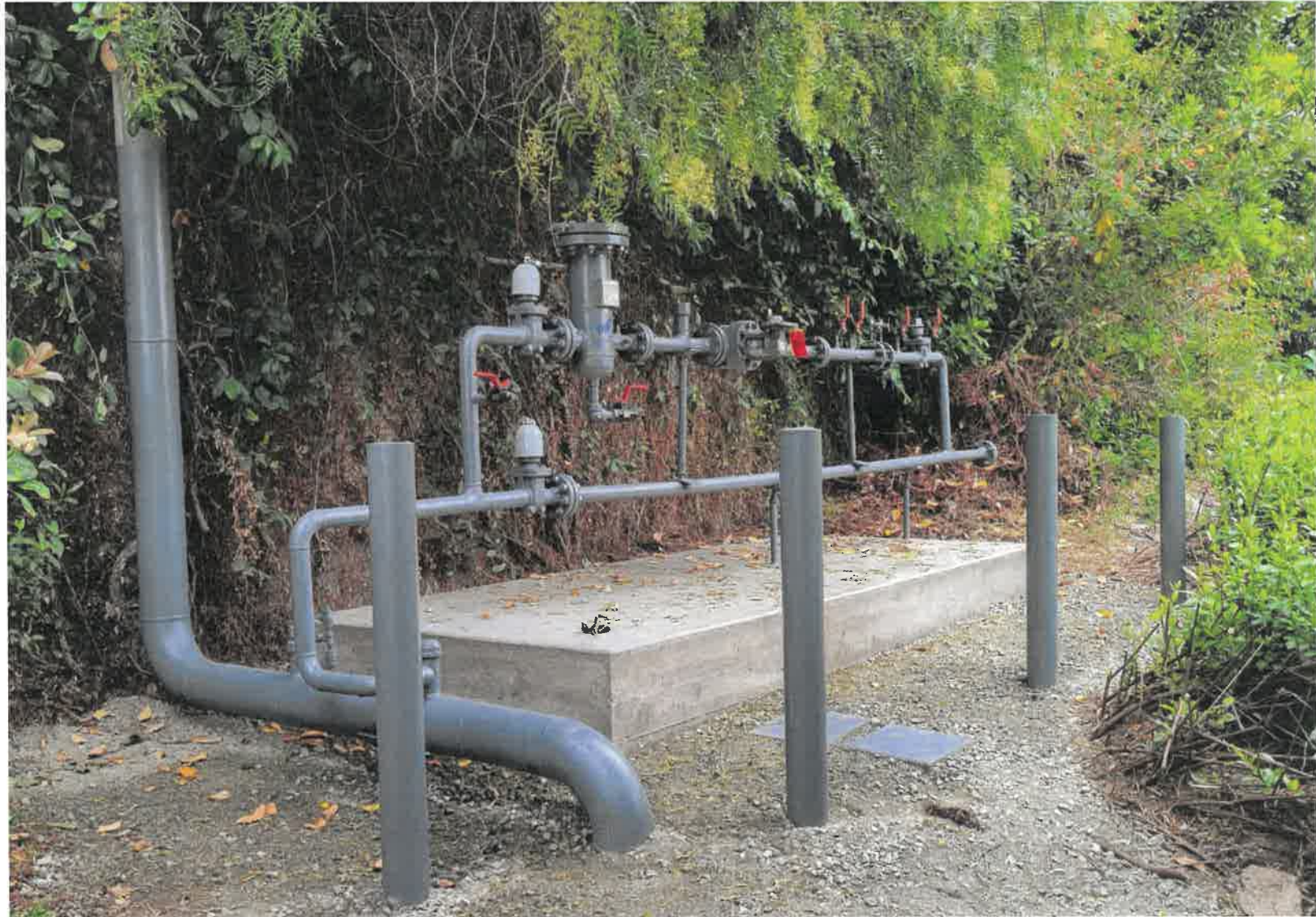
Figure 1 - New gas meter set assembly installed over concrete pad in the parkland (4/13/2021)
