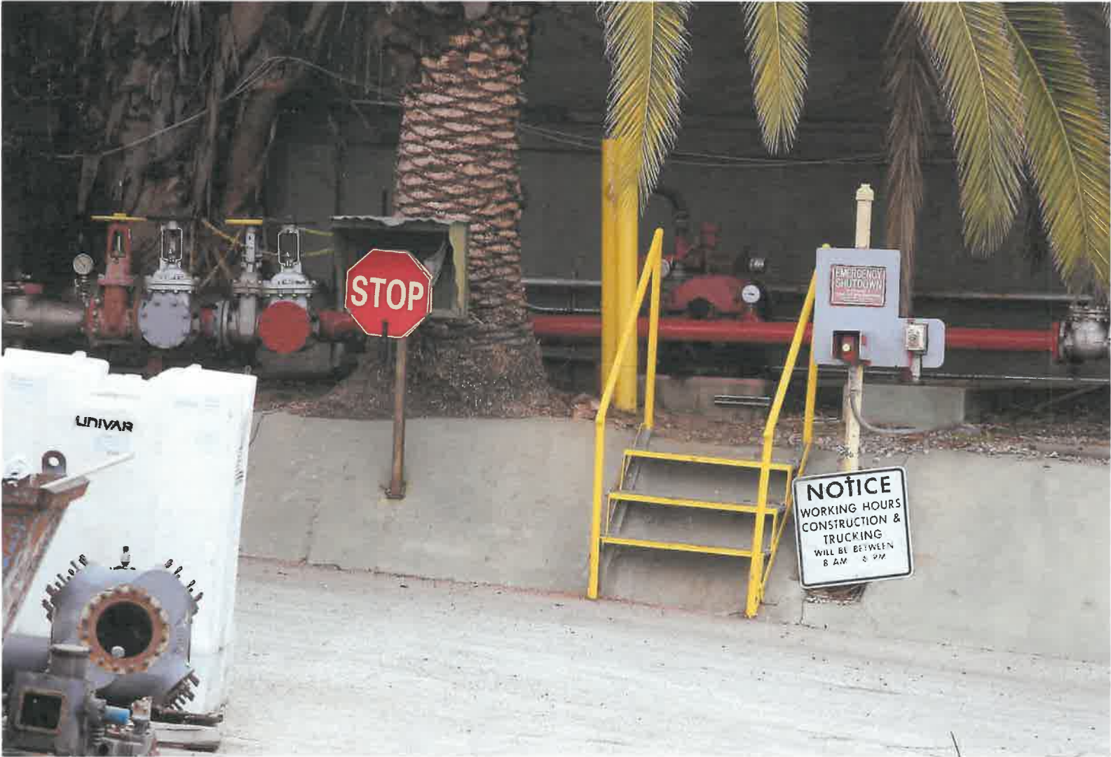
Figure 14 - NOTICE WORKING HOURS AND CONSTRUCTION & TRUCKING WILL BE BETWEEN 8 AM - 6 PM
