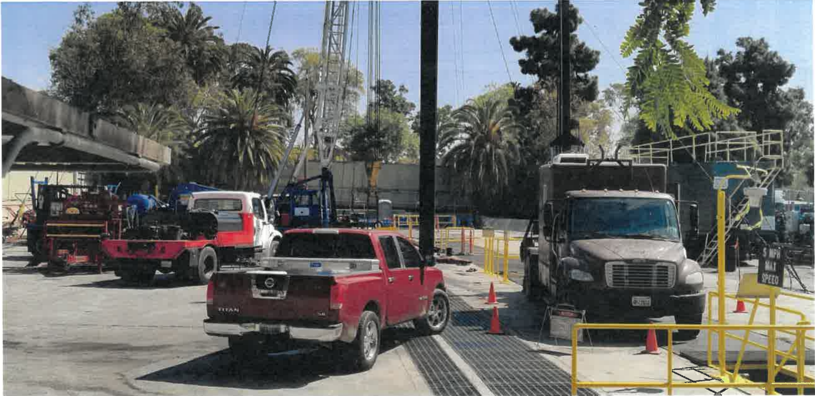
Figure 33 - A dirty, brown PDI trucked equipped to use radioactive materials parks on site (3/18/2021)
