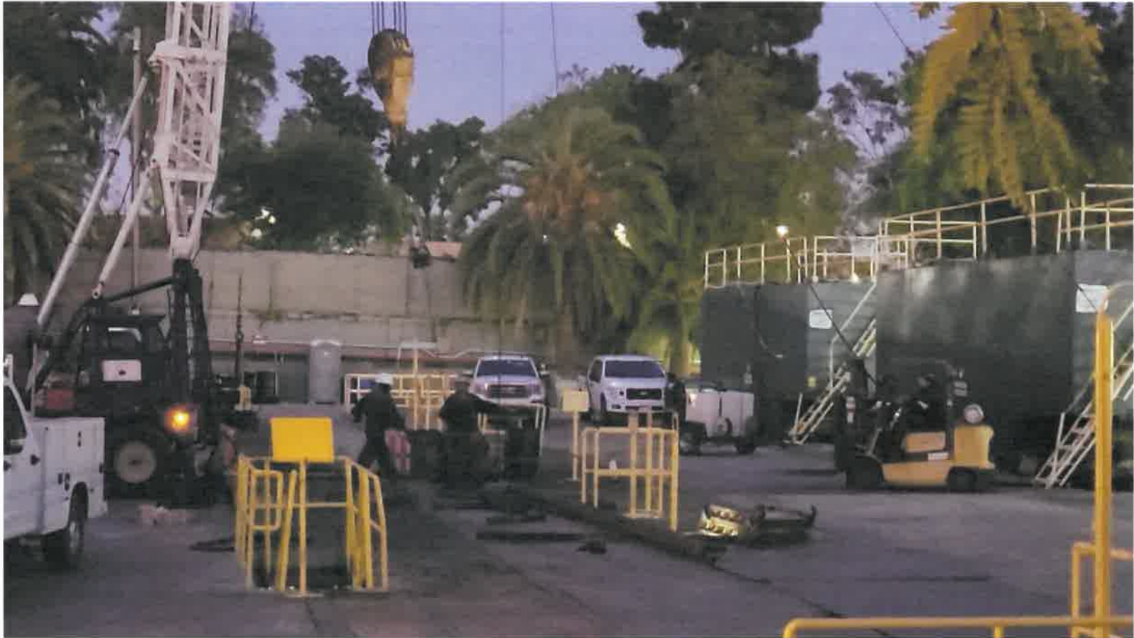
Figure 12: The workover rig lowers a heavy valve guided by a forklift and two workers in the dark (3/26/2021)
