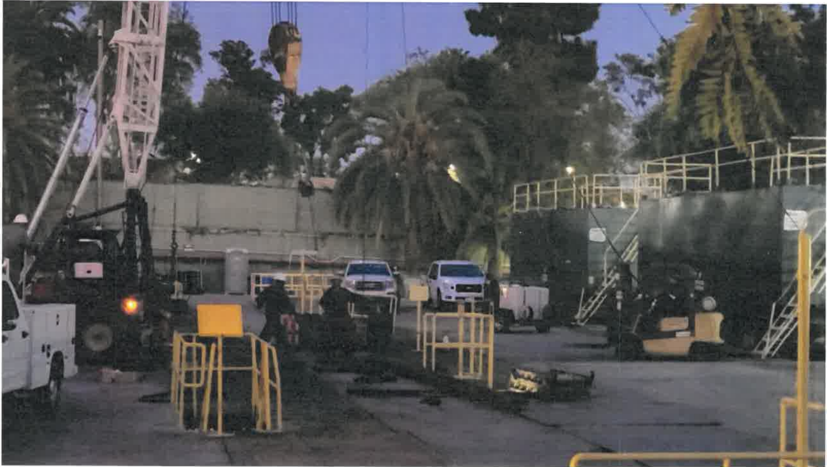
Figure 12: The workover rig lowers a heavy valve guided by a forklift and two workers in the dark (3/26/2021)
