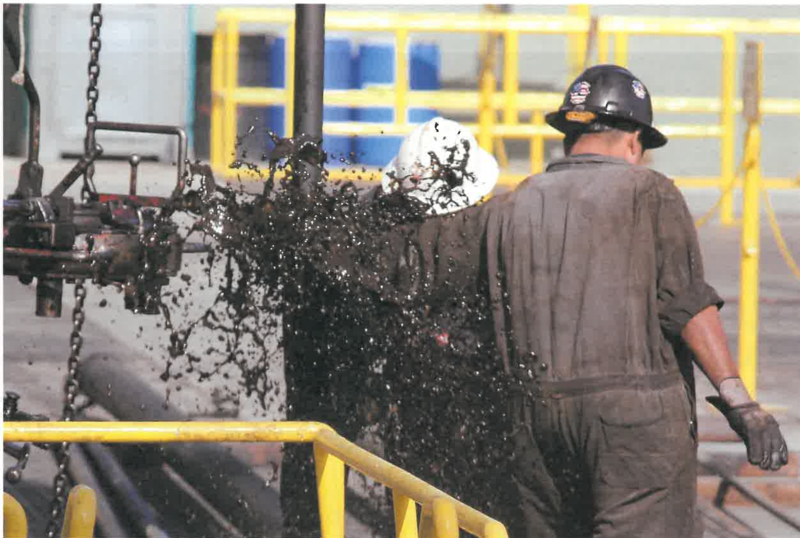
Figure 26 - Oil splashes bare armed workers who tried to suppress the oil burst by wrapping the pipe with a plastic trash bag (4/15/2021)
