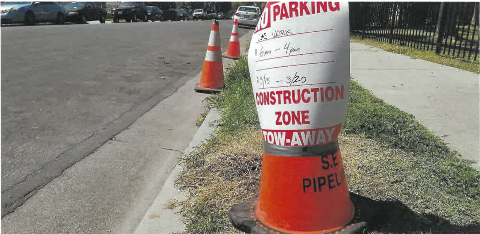
Figure 7 - - Fake NO PARKING / TOW-AWAY zone created by workers at Murphy on 27th Street (3/17/2021)
