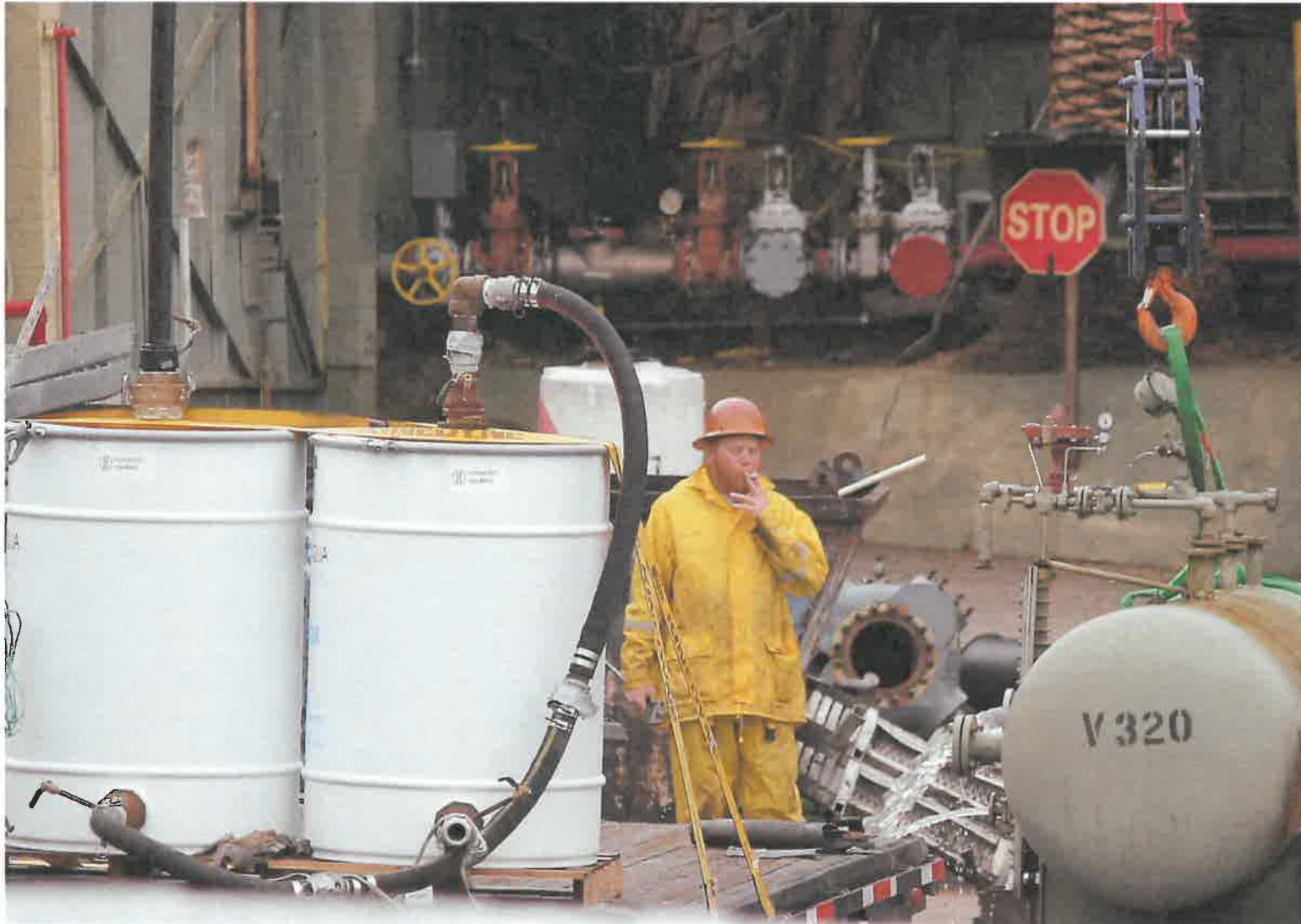
Figure 28 - Worker smokes on the drill site (3/15/2021)
