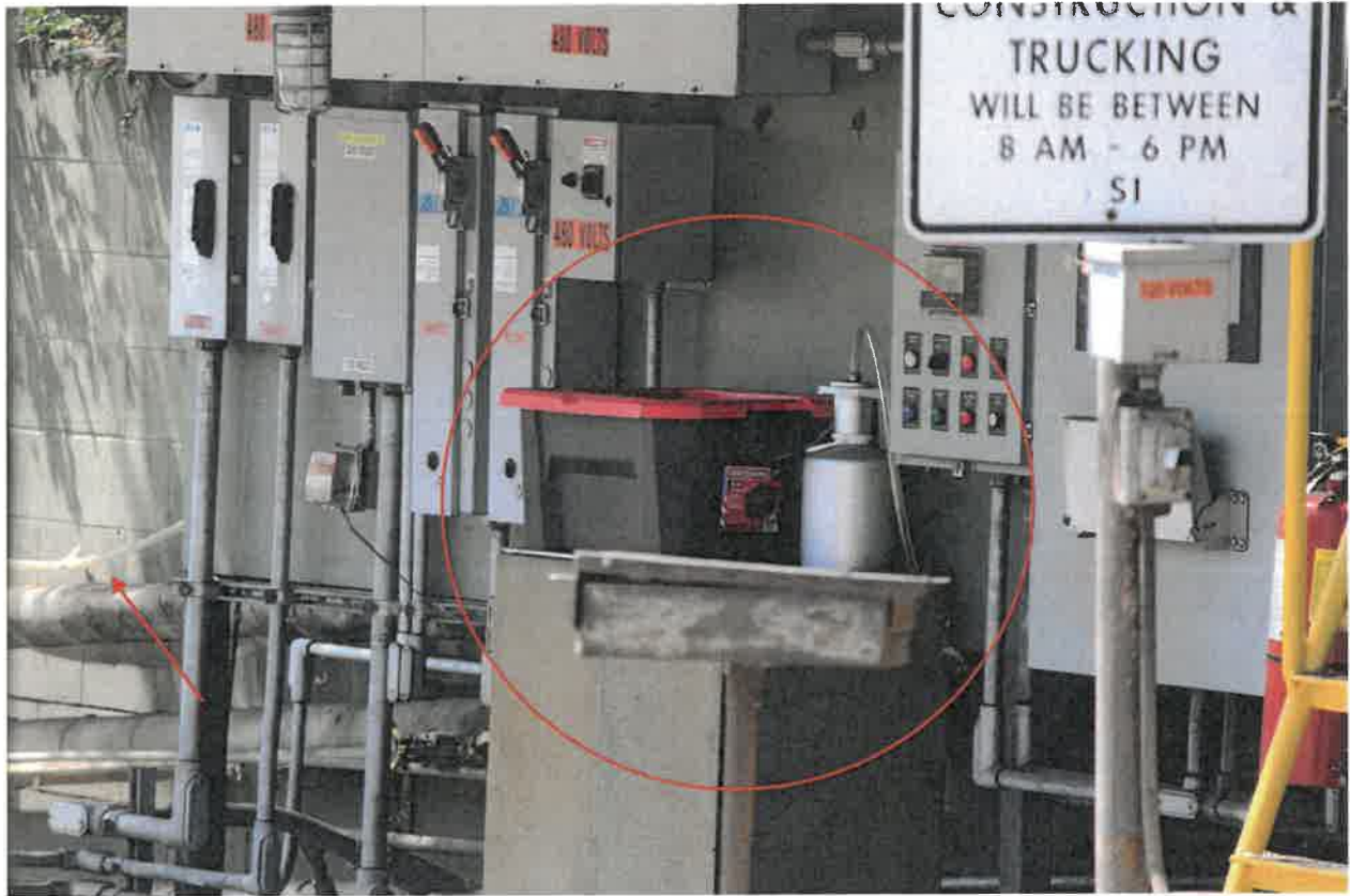
Photo 5: The silver device appears to be a diffuser for dispersing odor counteractant. A clear plastic tube emerges from the top, runs under the shelter and then along the wall shared with the AIDS Healthcare Foundation. The device appears to be connected to the black plastic bin by a white tube.
