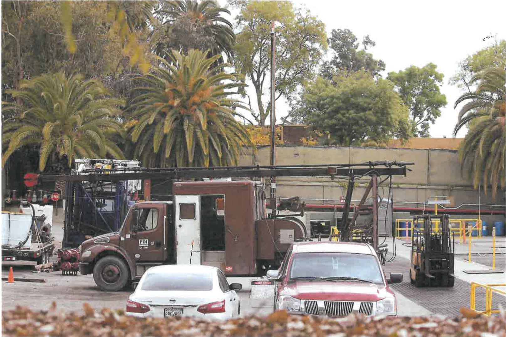
Figure 36 - The PDI truck returned to the drill site again setting out a warning sign (between vehicles) warning that radioactive materials were in use (3/25/2021)
