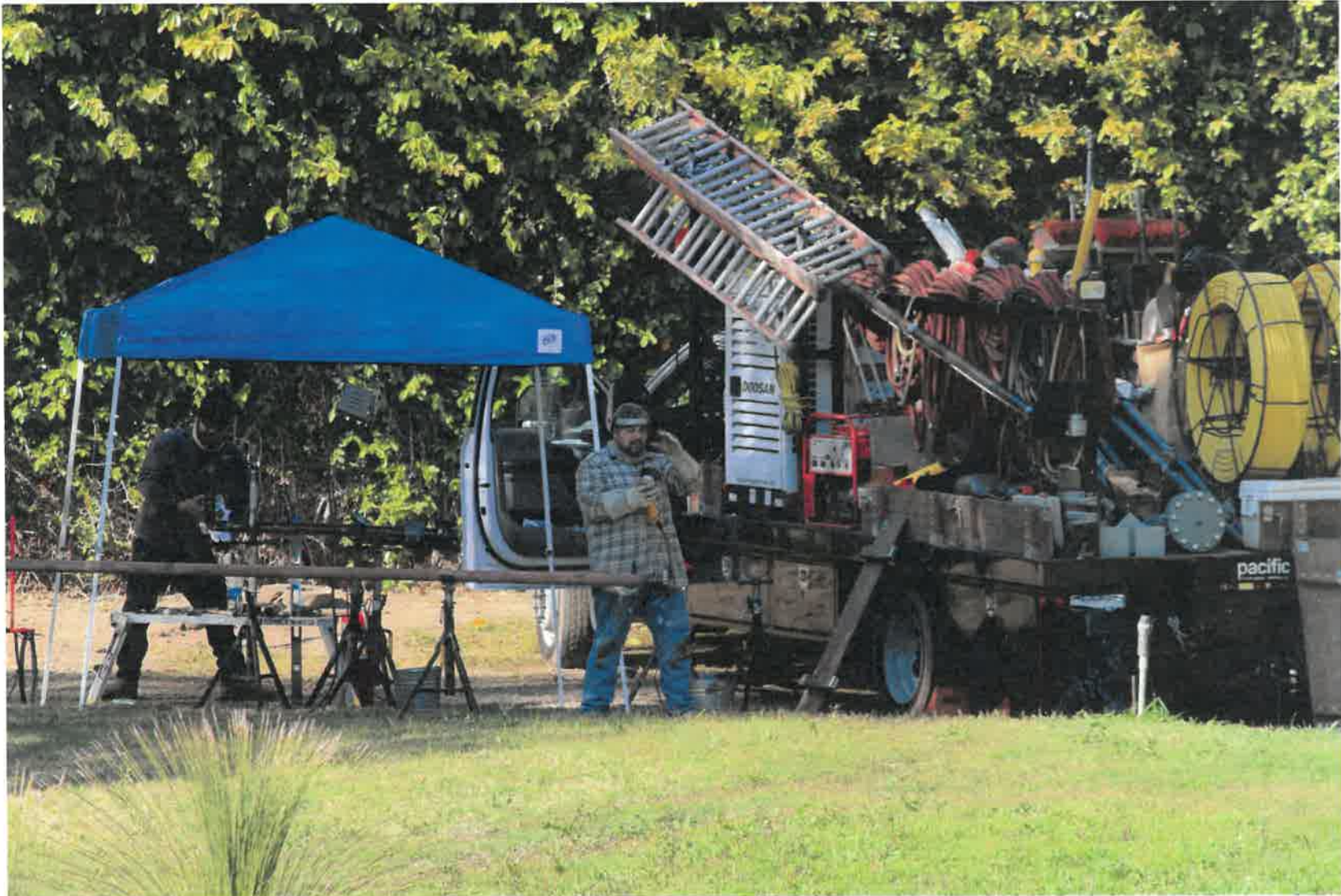
Figure 3 - Trucks and tents in the parkland. Pipe fitters and welders build a new gas meter set assembly (March 19, 2021)
