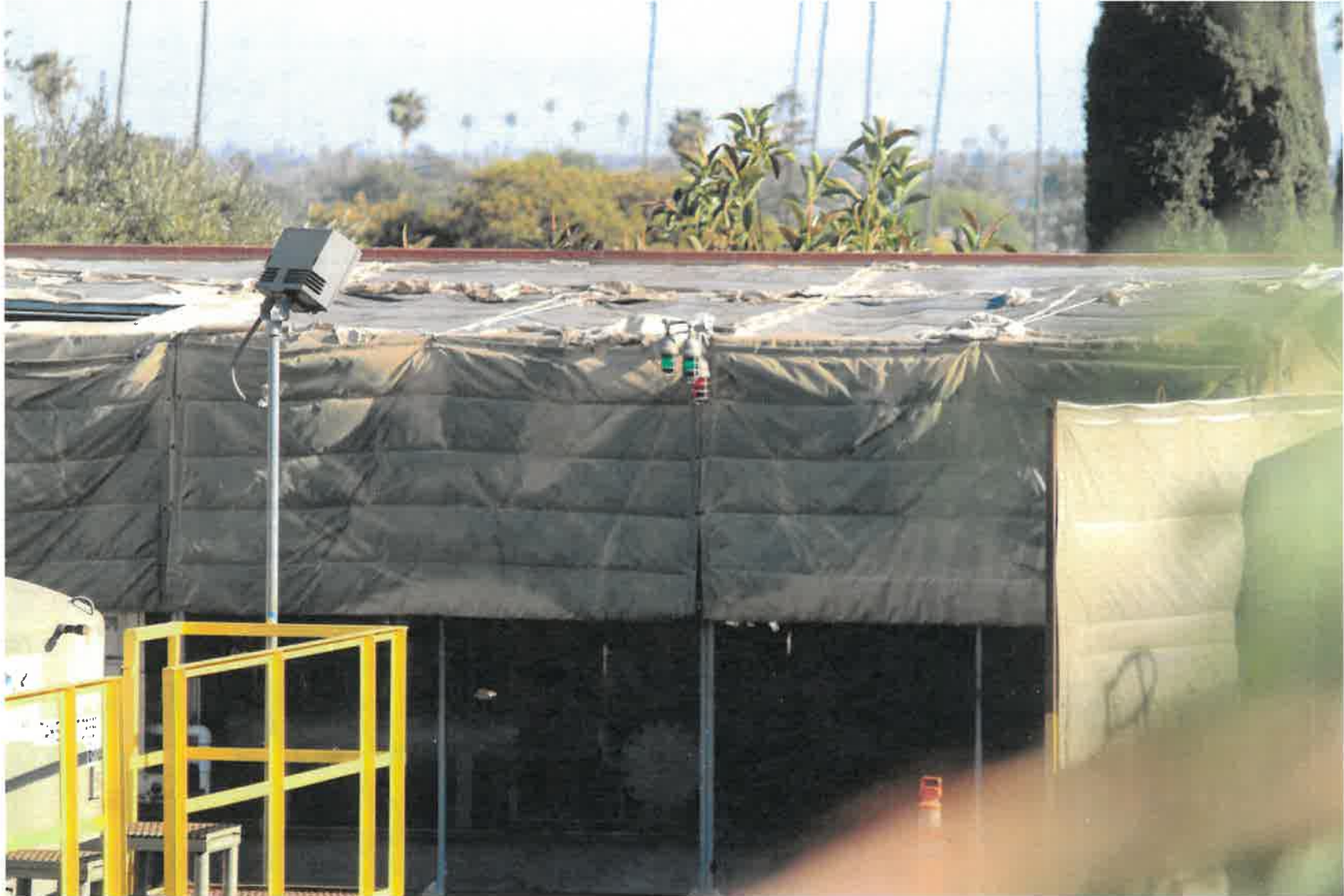
Figure 17 - Dilapidated sound blankets in the southwest corner of the drill site next to the AIDS Healthcare Foundation building.
