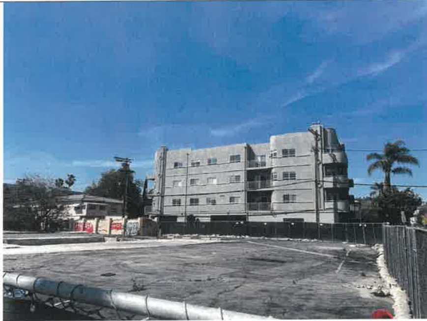
7. Taken from the SE corner of the project site, NW into the project site.
