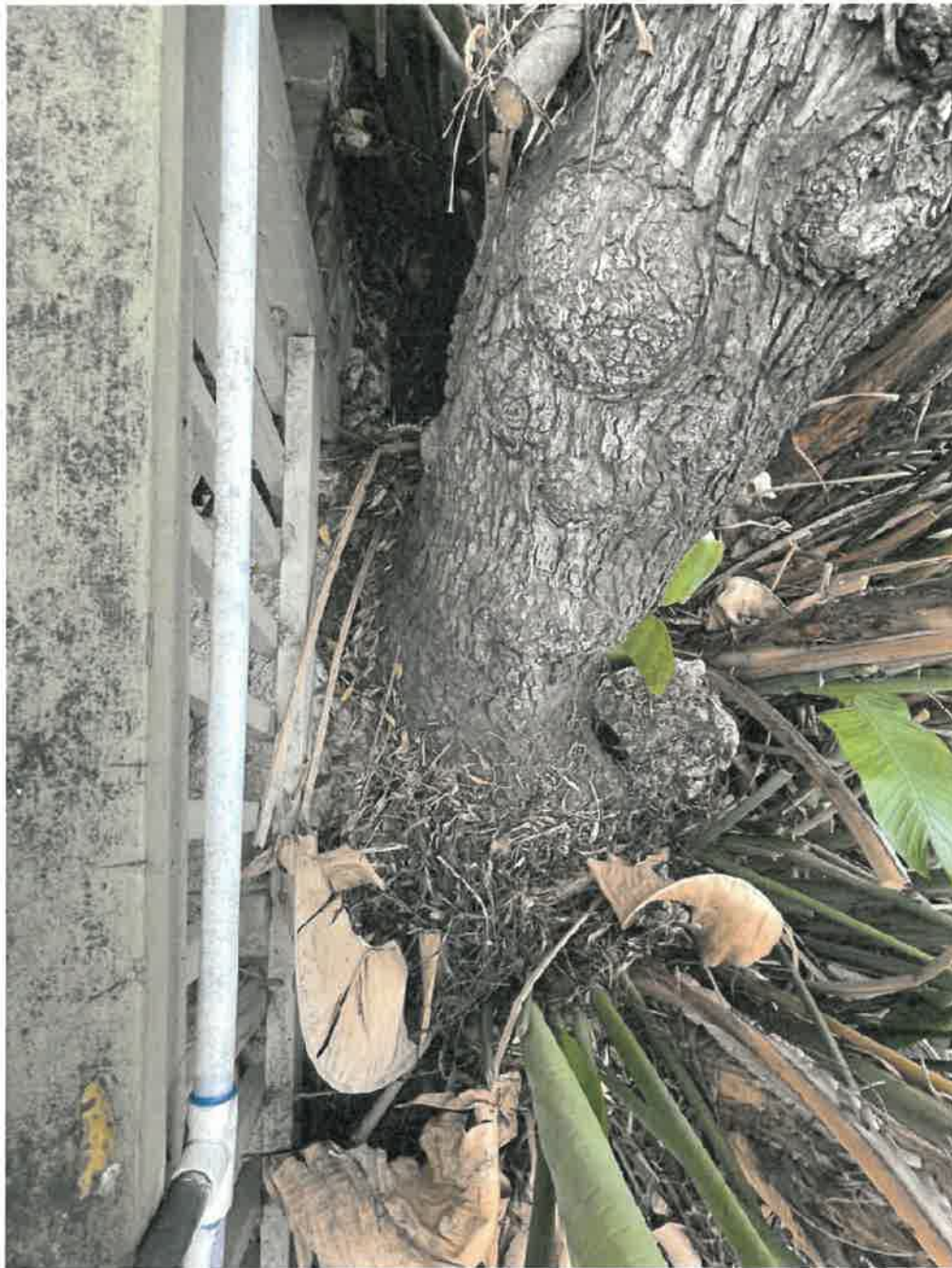
PHOTO 3 - Note the restricted space. Concrete is cracked at the base of the trunk on the right side, where the edge of the vintage wall is located.
