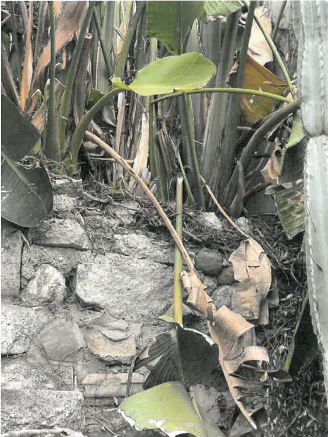
PHOTO 5 - Vintage concrete planter wall in front of the black walnut tree. This wall must be removed and remediation performed for this steep slope.
