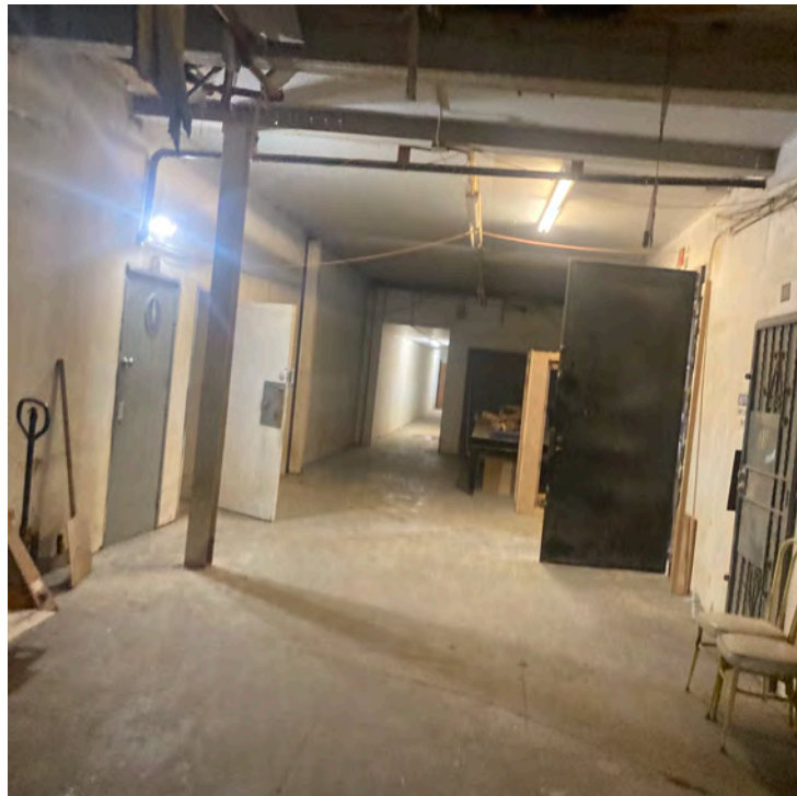
First floor hallway inside Cadet Records showing where record presses, recording studio and other equipment were located. 2023 (J. Kress)
