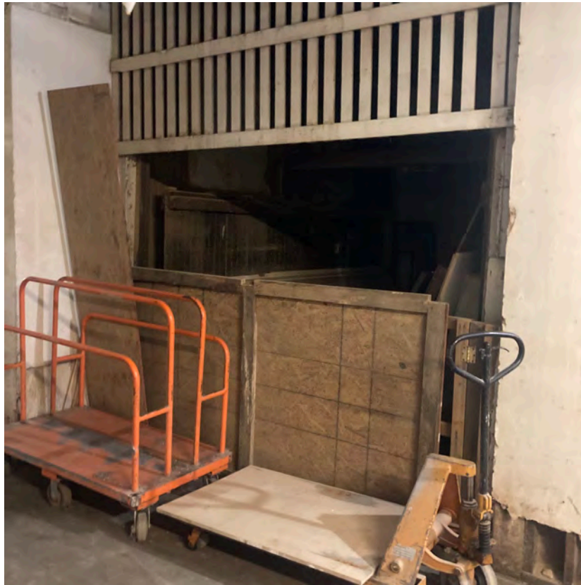
Freight elevator inside Cadet Records. 2023 (J. Kress)
