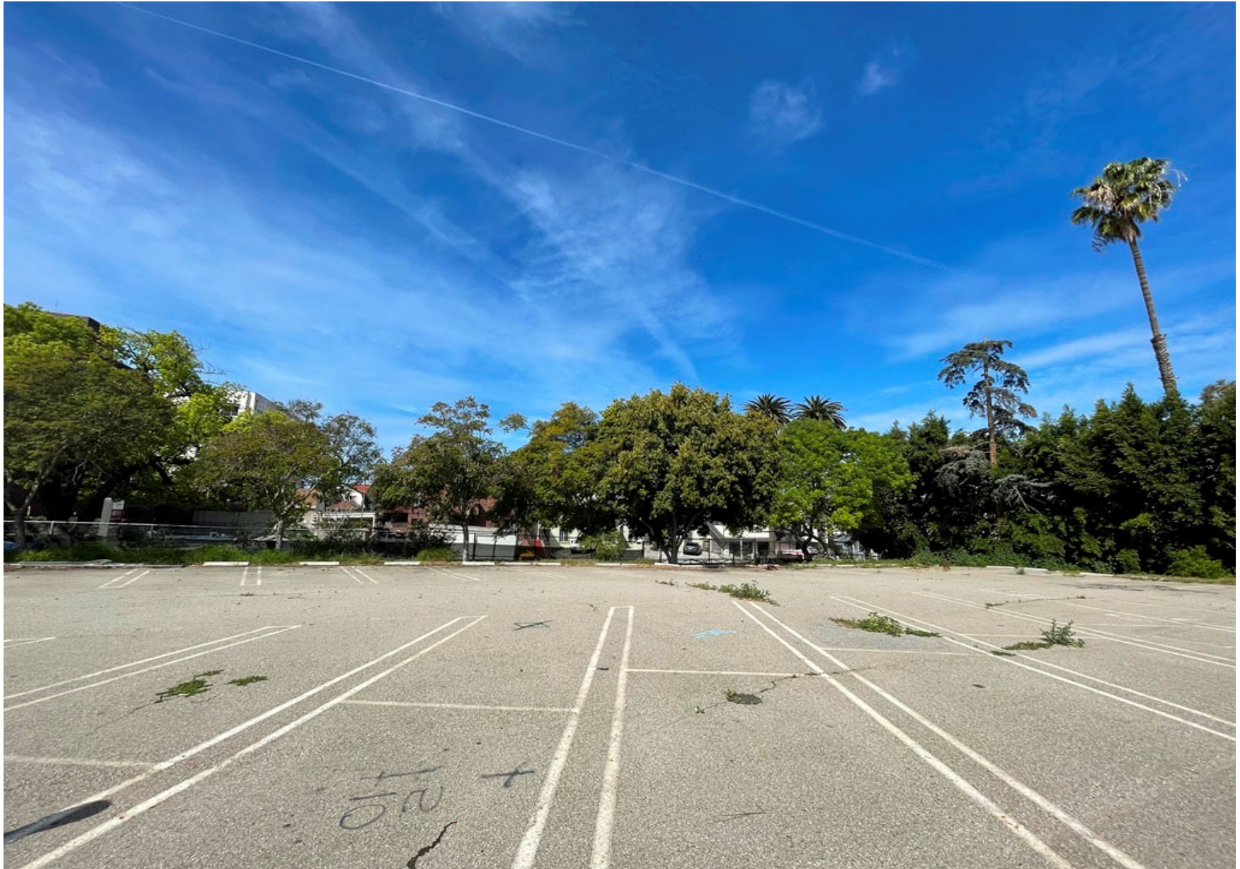
West edge of the parking lot on Gramercy and trees #8 to 17 from right to left.
