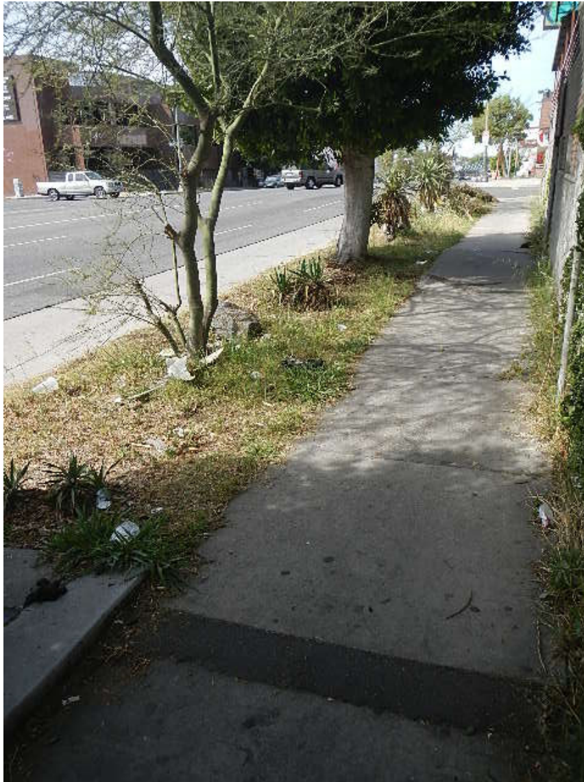
#4 Indian laurel and sidewalk lift
