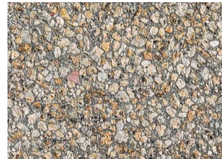
CIP CONCRETE PAVING TYPE 1 BROWN INTEGRAL COLOR CONCRETE W EXP AGG FINISH
