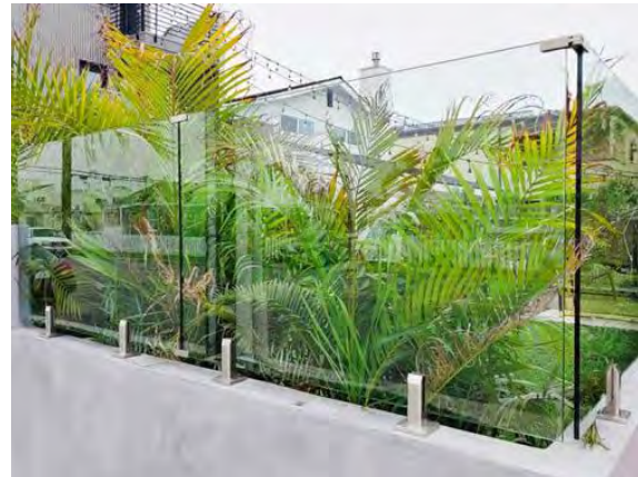
GLASS GUARDRAIL (POOL ENCLOSURE)
