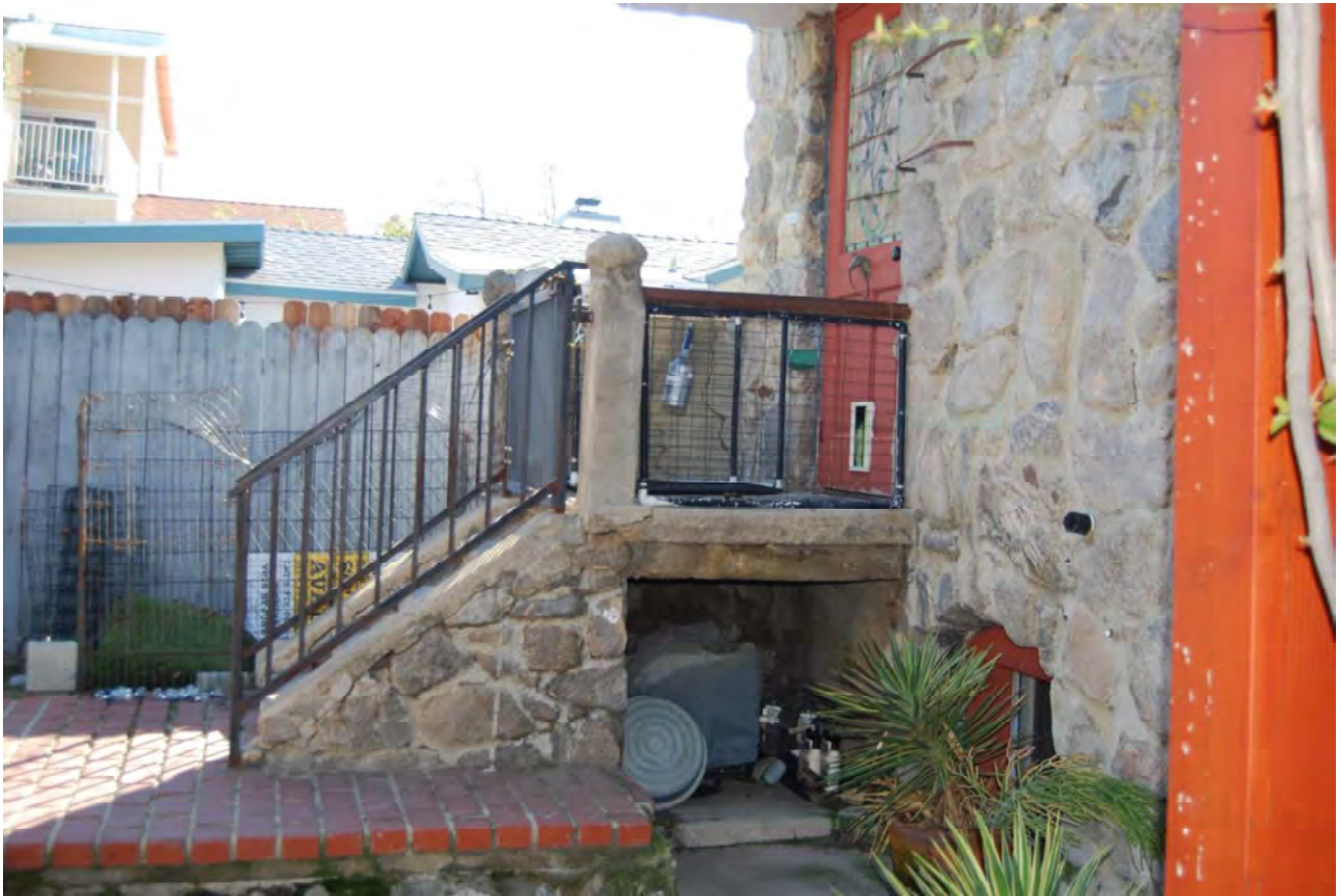
Elmer Reavis House, rear steps, 10620 N Samoa Avenue, January 24, 2023, (Photograph by Charles J. Fisher)
