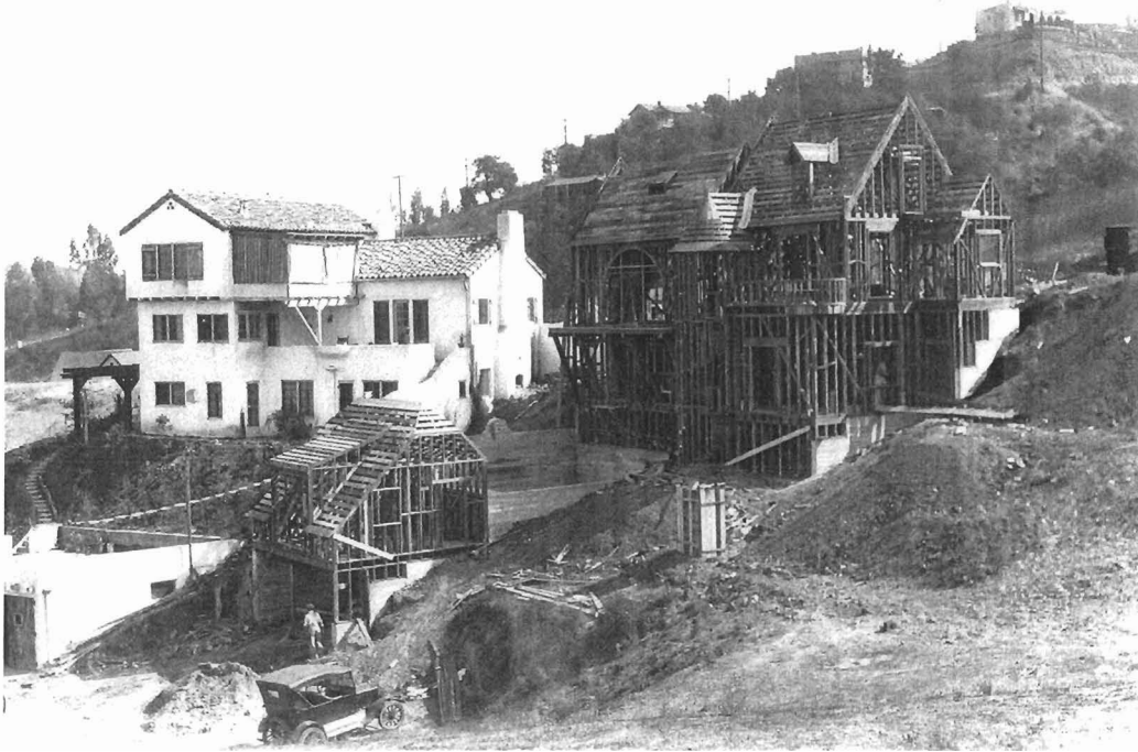
Garage, guest house and residence under construction: Viewed to the southeast. Photo source: Estate of R. E. Hill ~ Date: 1927 ~ Photographer: R. E. Hill.
