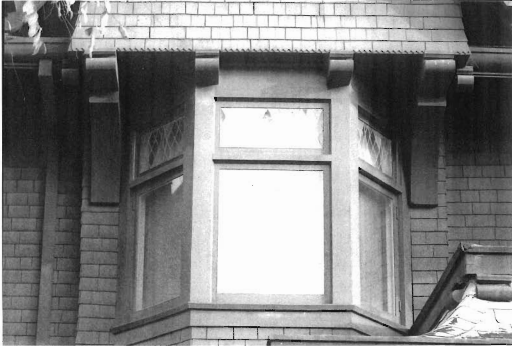
West façade second story slant bay window of master bedroom; fixed transoms with multiple leaded diamond lights over single lights, viewed to east. Note decorative shingle finish course, above.
