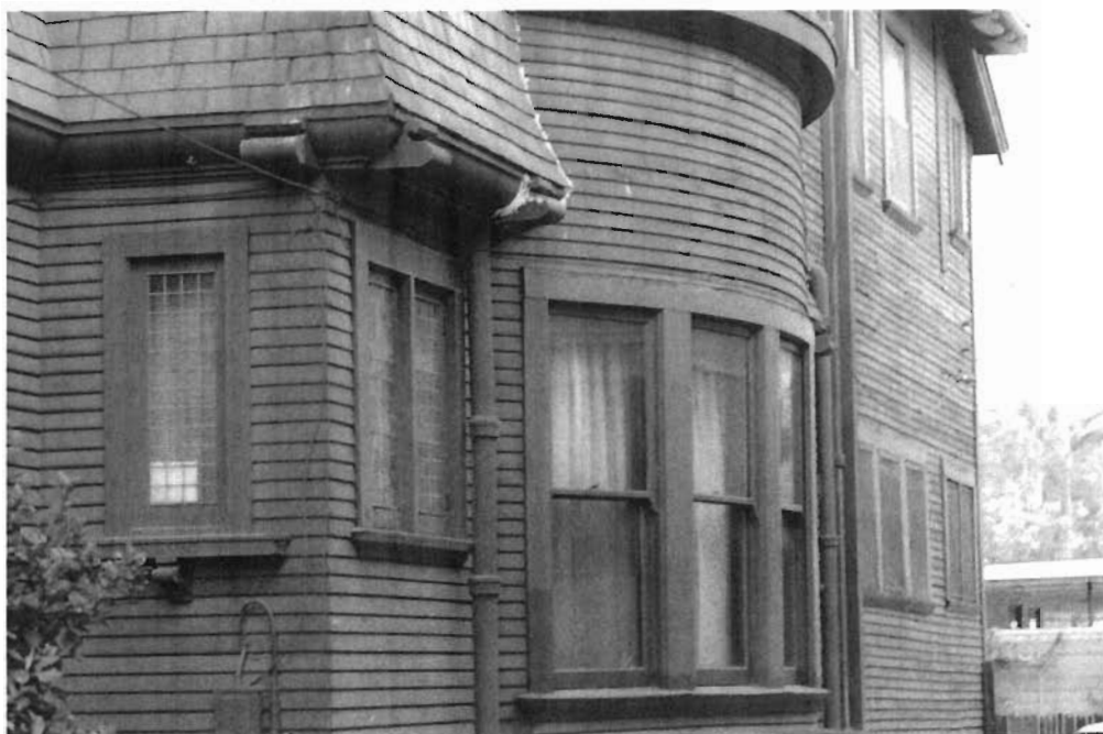
Residence southwest corner, curvilinear dining room bay, south elevation, viewed to northeast.
