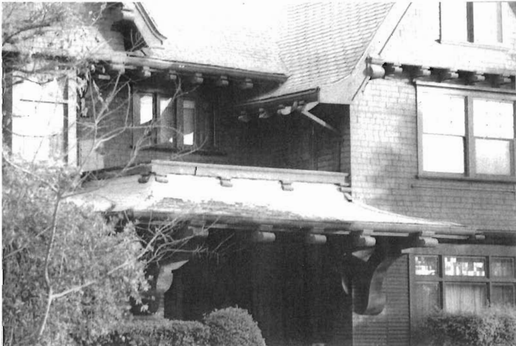
Projecting entry porch roof and second story recessed porch, viewed to southeast. Note decorative rafter tails and brackets.
