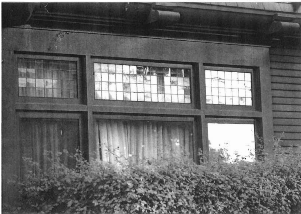
West façade library triptych windows with multi-pane leaded glass fixed transoms over single lights, viewed to east.
