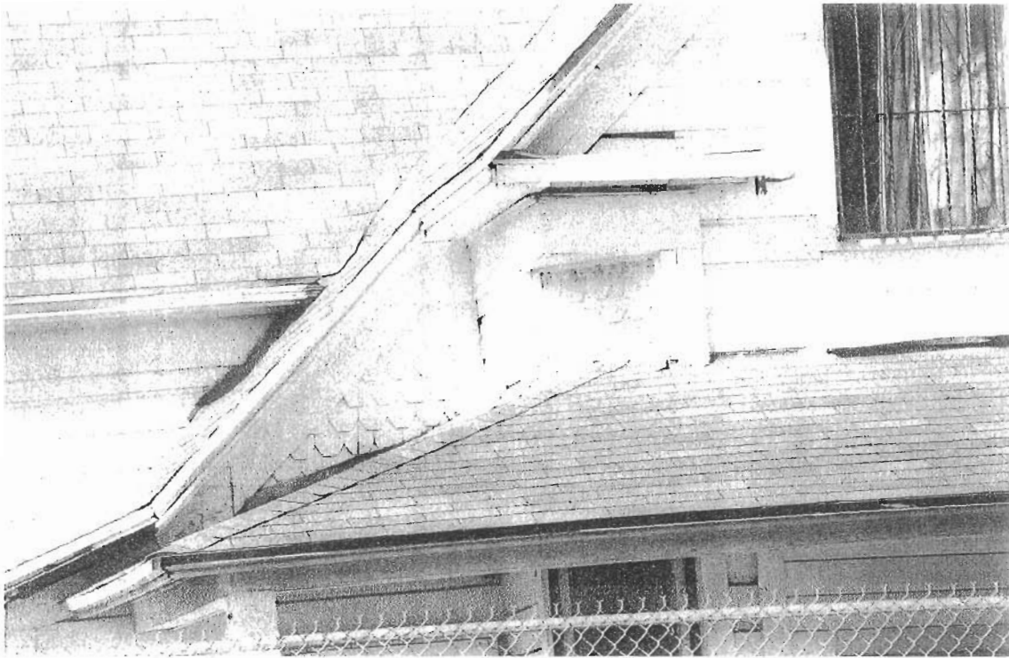
East façade gable end and gable projection with fish scale shingle detail.
